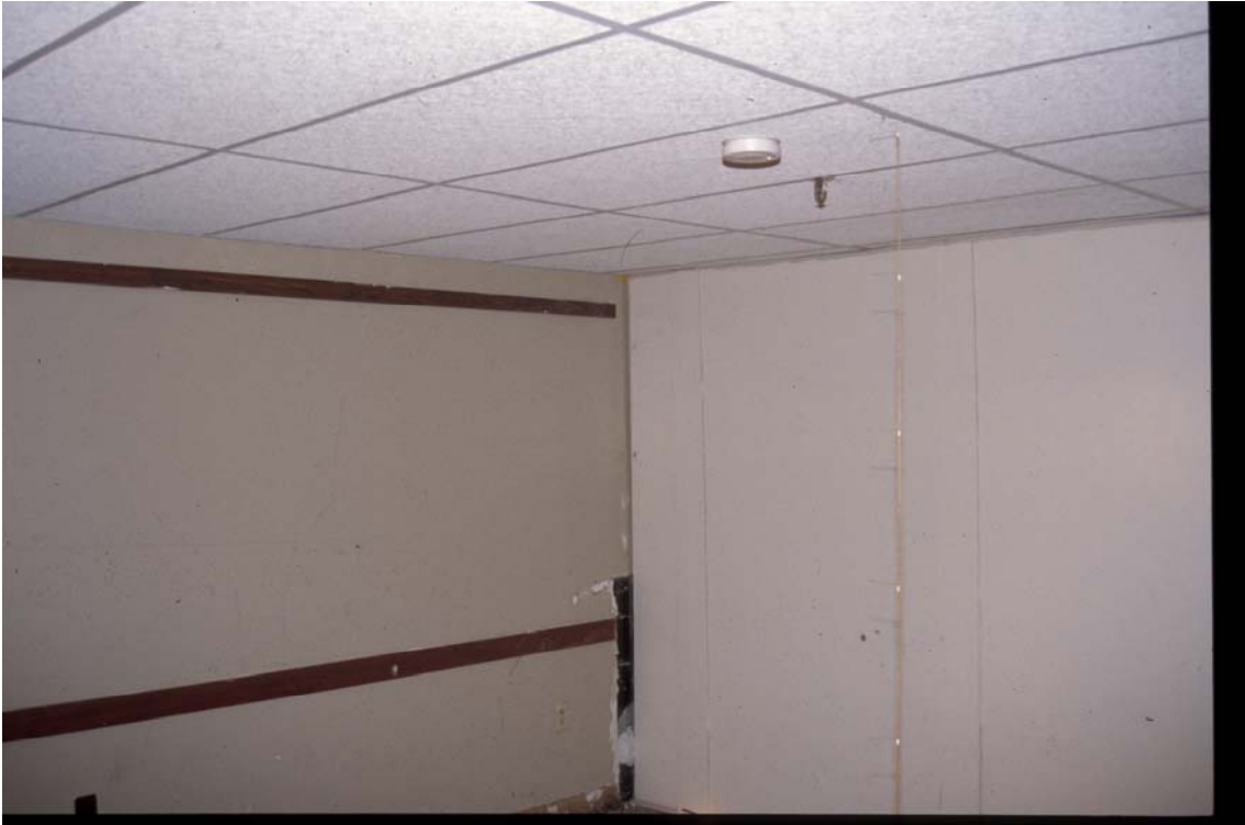
Figure 4. Photograph showing ceiling tile
