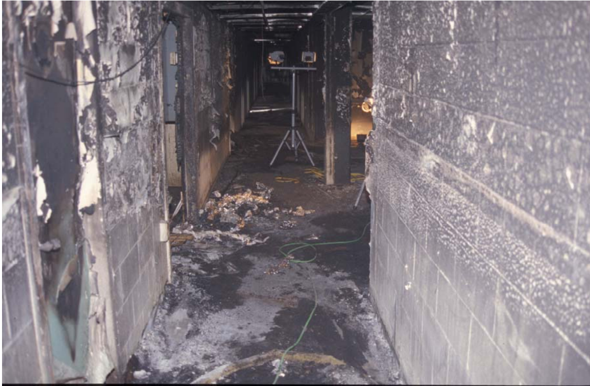
Figure 16. Photograph of corridor from the west approaching day room on right, after experiment 3.
