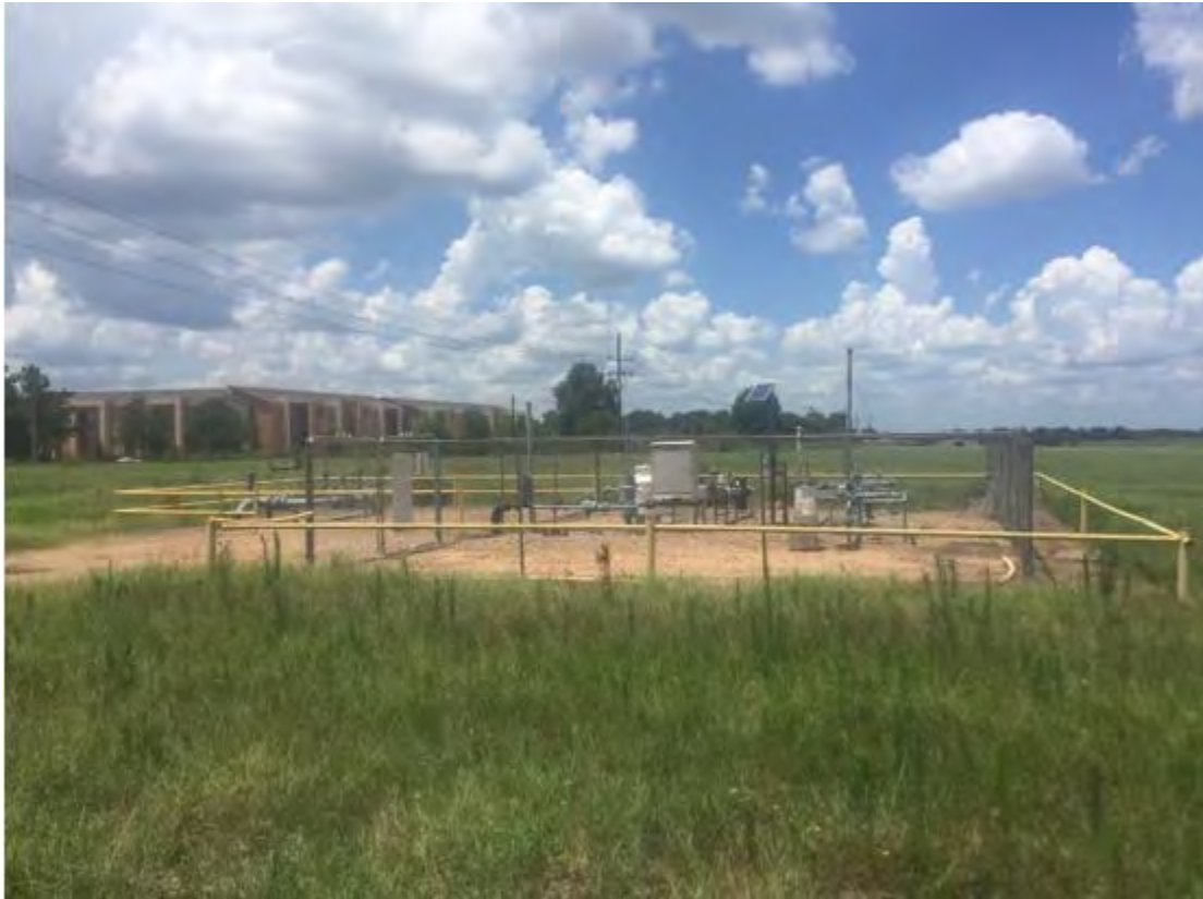
Figure 9-2: Existing Gas Metering Station
